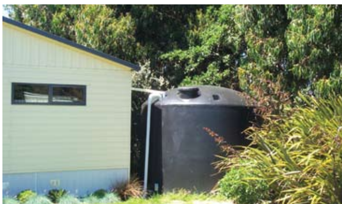
Polyethylene rainwater tank at a school in rural Auckland.
